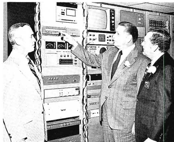
5-million watt ribbon-cutting. Official turn-on for WTAF-TV's new transmitting plant is handled by Philadelphia Mayor Frank Rizzo. Looking on are Neil Vander Dussen (left), Division Vice President, RCA Broadcast Systems, and Bob Weigand (right) then General Manager of TV-29, and now Taft Broadcasting Company Corporate Vice President.
